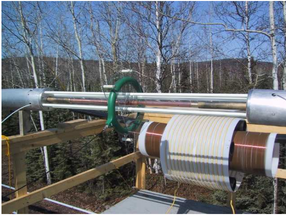
Fig. 2. Center of the 2.85-MHz Hertz dipole, seen in Fig. 1, showing the self firing pressurized SF 6 spark gap, Tesla primary and secondary antenna charging coils, and green antenna current monitoring transformer, surrounding the electrodes of the spark gap.
